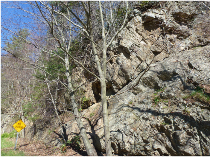
Figure 6: Potential rock-slide detachment surface (visible from bottom-left corner to top-right corner of image) created by intersection of foliation and fractures.
