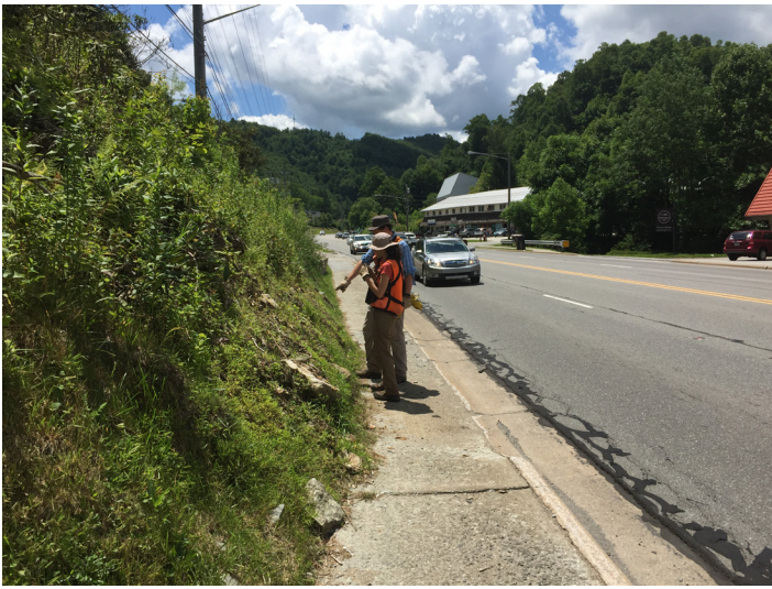
Figure 9. Photograph of the rocky debris at the slide toe impinging on the sidewalk along SR 105. View looking west. 2018_07_05 NCGS photo.
